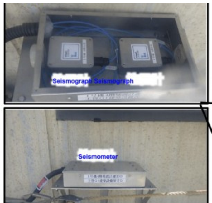
Seismometers at unit 1
