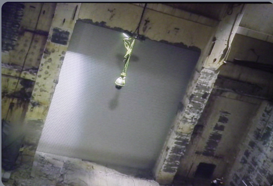
Images above, unit 2 refueling floor exterior wall before and after cutting to install an overhead door.
