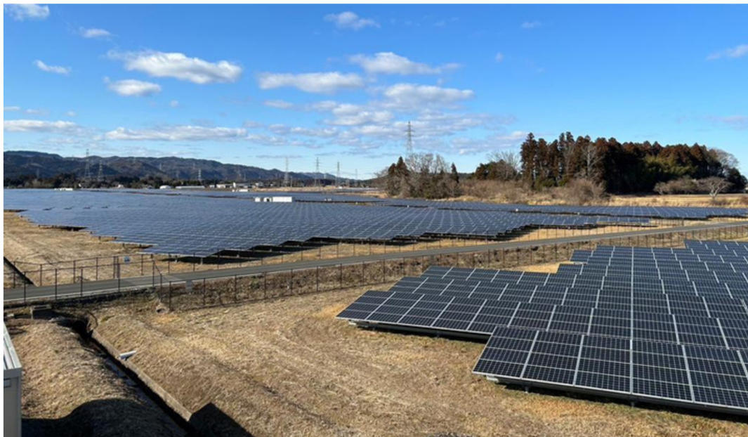
Image above: Solar panels installed on farm fields in Tomioka, Fukushima Prefecture Image credit - Saki Kobayashi
